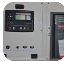
Control Panel & MCB
